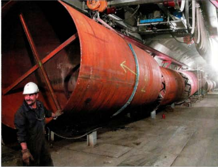
Construction: the assembly in the target chamber of the 6 m long sleeves into 18 m long sections of the decay tube.
