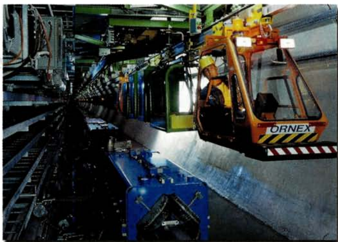
One of the monorail trains suspended from the ceiling above the magnet ring in the 27 km long LEP tunnel. The trains were used for transporting goods and people.
