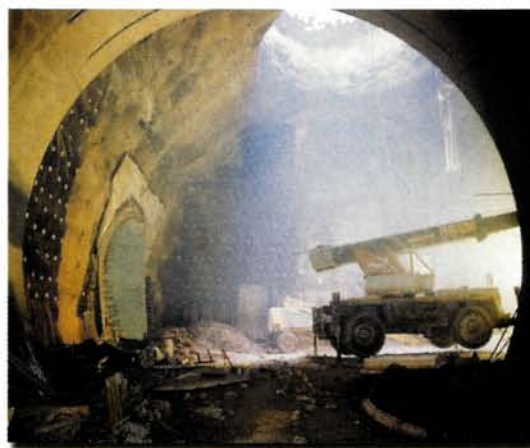
In 1985 excavation work began for the 27 km tunnel of the Large Electron Positron collider (LEP). This was the most formidable civil-engineering venture in the history of CERN and Europe's largest civil-engineering project prior to the Channel Tunnel.
