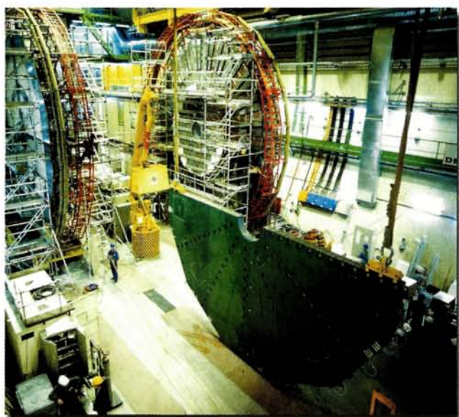
The construction of DELPHI, one of the four detectors at LEP, in January 1989, only seven months before the first collisions. This picture shows the installation of a "half-moon" section for one of the end caps.
