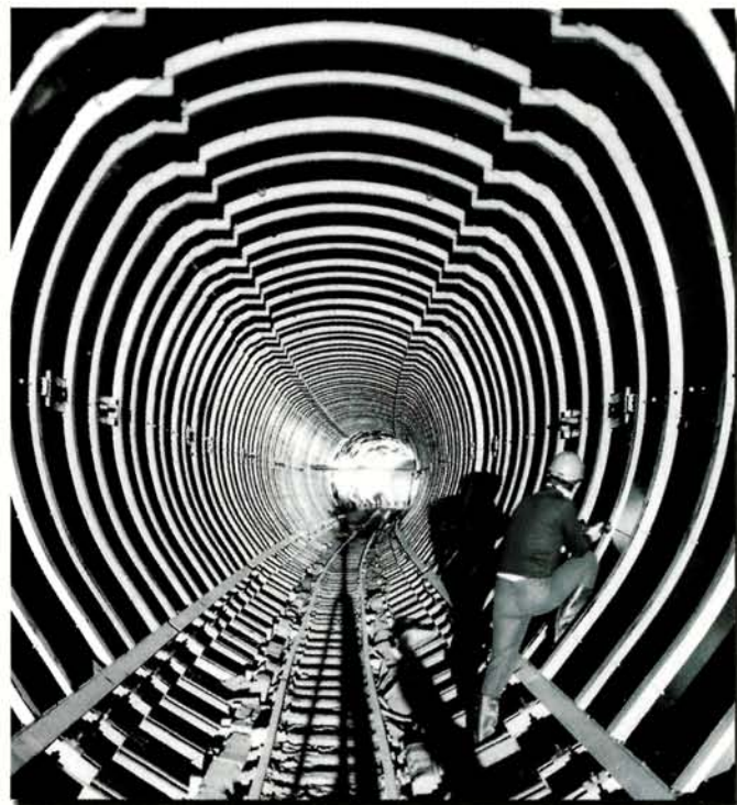
The SPS, with its 7 km circular tunnel, extended CERN beyond the Meyrin site. Construction began in 1972. Here the metal structure of the shuttering used when pouring the concrete walls of the tunnel gives a remarkable optical effect.
